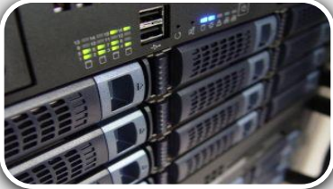
Server side networking
