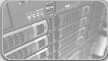
Server side networking
