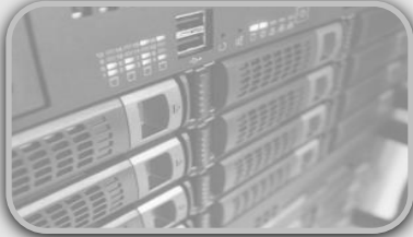
Server side networking
