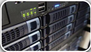
Server side networking
