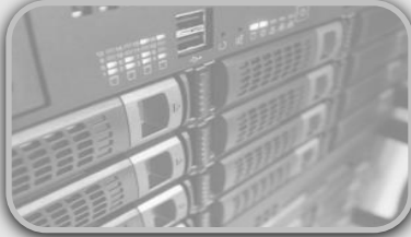
Server side networking
