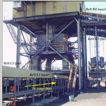
Figure 1: A critical transfer station at DBCT which was modelled using discrete element analysis and HPC.
